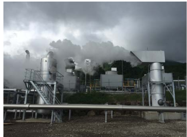
Geothermal power plant facilities near the Beppu
